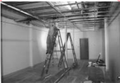
Brian Grubbs, office manager, hanging ceiling grid in the new collections storage area. In order to save substantial costs, the Museum utilized its own internal labor to complete practically all construction on the project.
